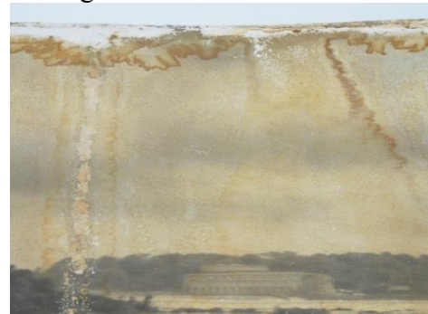
Fig. 8. Overall staining caused by humidification
